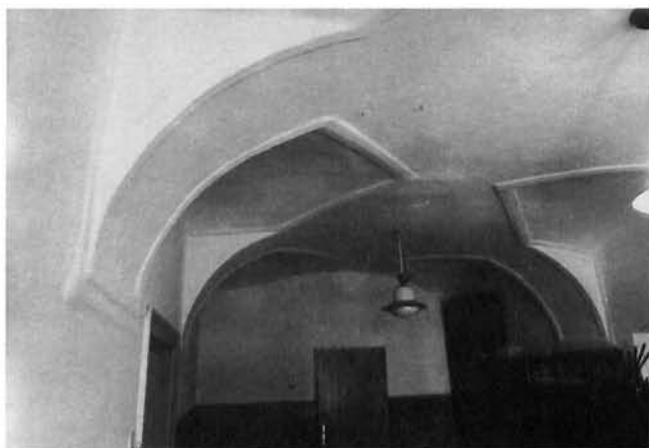
Svod u prostoriji prizemlja (foto: Krešimir Tadić) Vaulting in the ground floor (Photo Krešimir Tadić)
