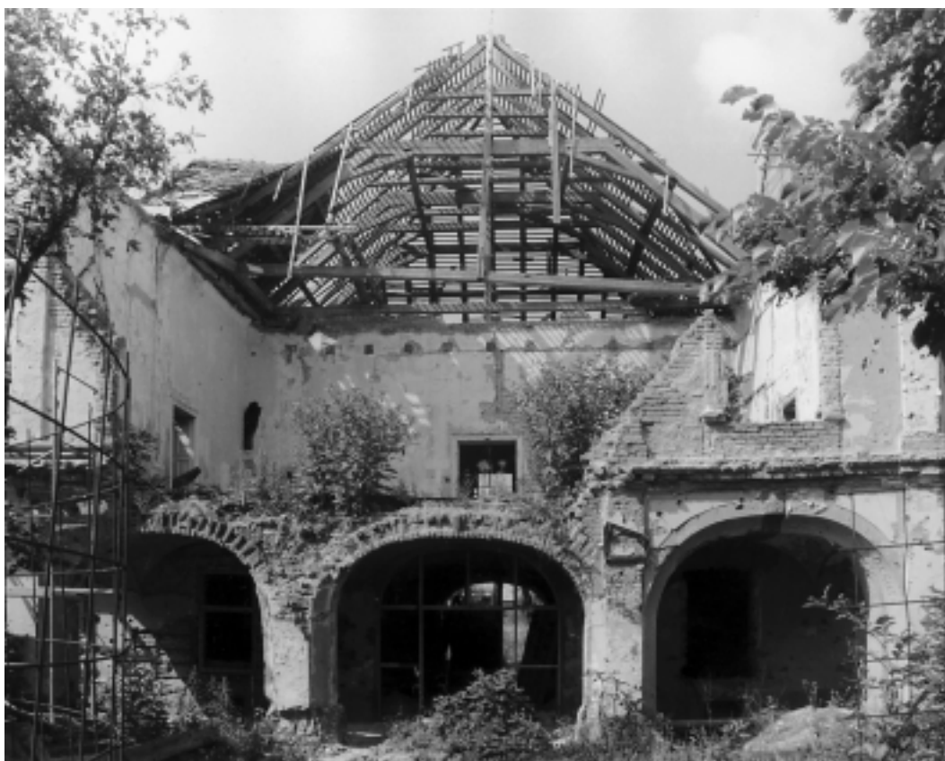
Županijska palača, urušeno pročelje, 1998. god. (foto: Milan Drmić) County Palace, caved-in front, 1998 (photo by Milan Drmić)
